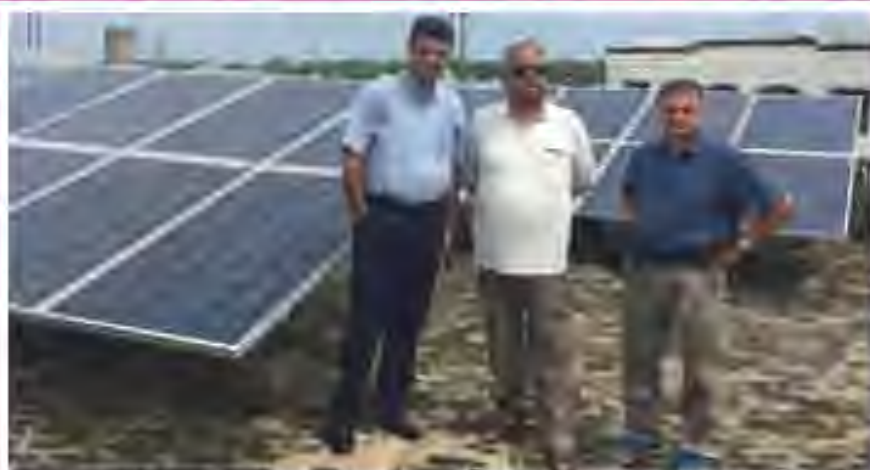
Sh. Shafiq Sultan, CEO, J K Energy Development Agency, Dr. Ajay Gupta, FIE; Chairman and Dr. H. L. Rawal, MIE; Hony. Secretary inspecting Solar Panels installed at The Institution of Engineers (India), Jammu Local Centre.
